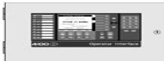
InfoAlarm Command Center in Remote Cabinet
